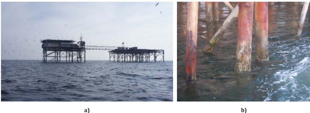
Figure 4 a) C-9 Baltic sea offshore platform, b) Damages of the supports of the C-9 Baltic Sea offshore platform
